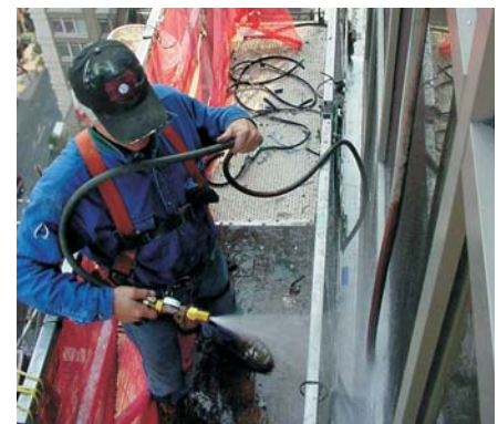
Field t est. following the AAMA 501.2 "Quality Assurance and Diagnostic Water Leakage Field Check of Installed Storefronts, Curtain Walls, and Sloped Glazing Systems" procedure.
